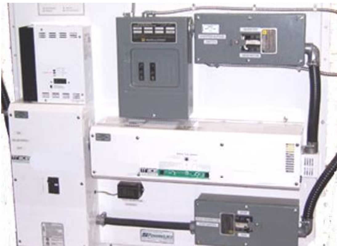
A typical installation with Solar PV Controller
