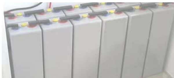
A gel-cell battery bank installed for a Stand-alone Solar PV System.
