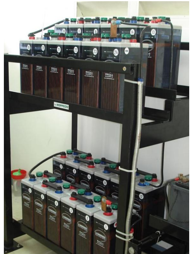
A battery bank used in a Solar PV System
